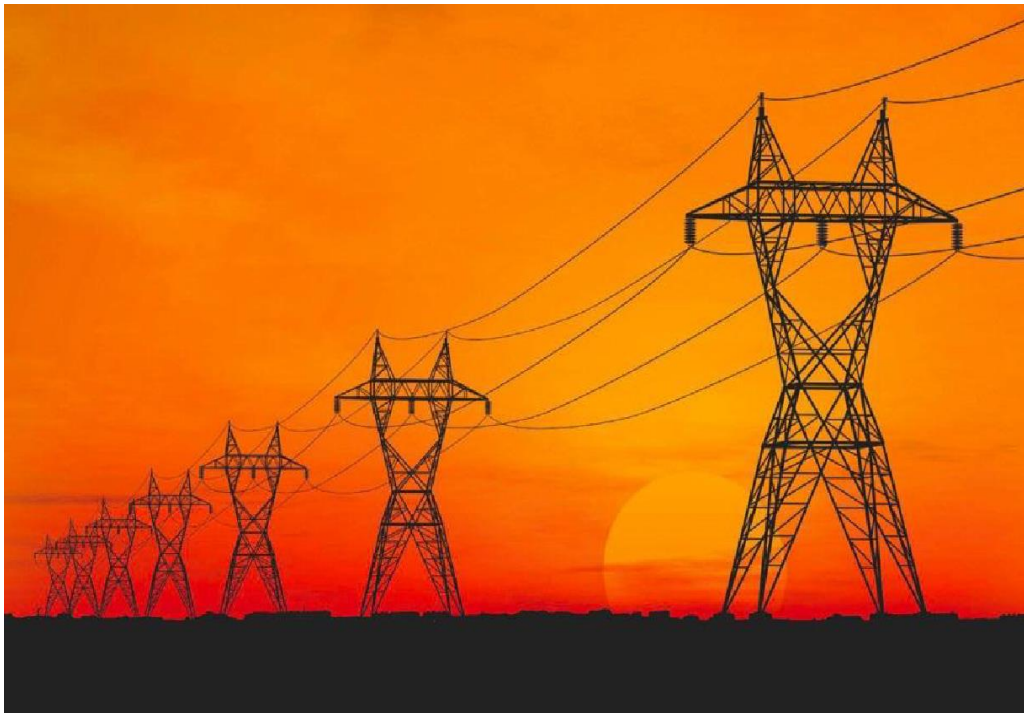
Figure 45. Ground wires in transmission lines
